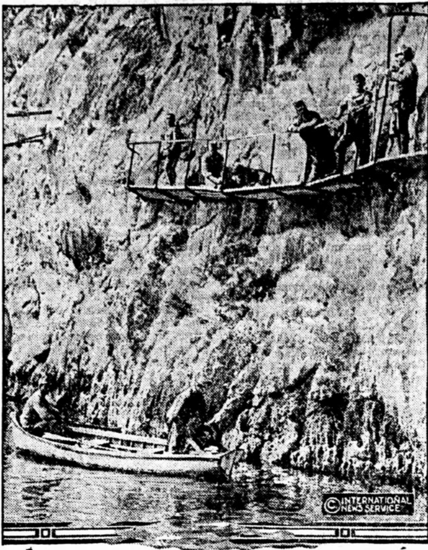
Austrian troops building a passway along the side of a mountain in the Tyrol to give them a new line for attack.
