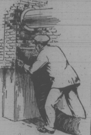
Removing Soot Accumulations From the Chimney is No Longer a Dirty, Messy Job. A Giant Vacuum Cleaner More Thoroughly Cleans the Chimney Than is Possible by Hand.
