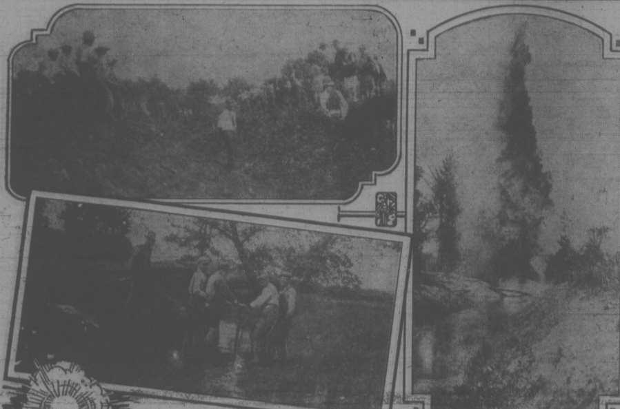
Blasting crew preparing to clean out an old ditch. Above—Adair County farm families view ditch they had seen blown by dynamite.
