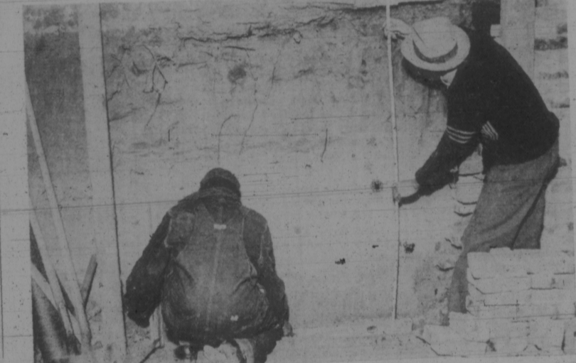
Arthur Turner is shown laying footing for the East Side Community center basement as Prezell Frazier takes
