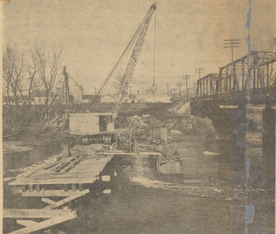
Because the S. W. Ninth street bridge over the Racoon river has not proved satisfactory for carrying telephone cables which serve much
