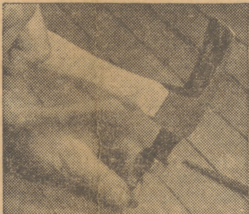
Sink protruding nail heads with hammer and nail set, then fill holes; eliminate squeaks by nailing to joist nearest the squeaks.
