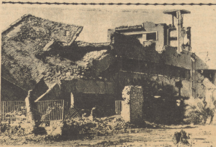
Above is a view of Suez City, which according to our Egyptian guides was completely destroyed for no apparent reason. Even the United Nations Building, the Mosques, hospitals, schools and Christian Churches were not spared.
