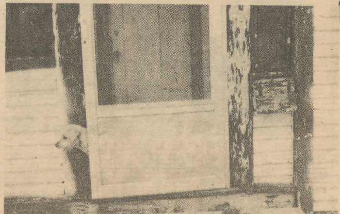
The front of the Williams house is badly peeling and easily accessible to any child in the neighborhood. The paint is easy to pick off and falls to the ground which makes it all the more available to little hands. And to make the frosting on the cake sweeter but deadly, its lead content is dangerously high.
