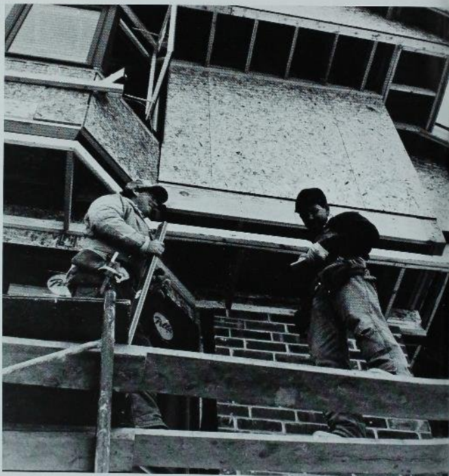
The new Alpha Tau Omega house is expected to be completed by Fall 1991. Construction workers Mike Tringham, left, and Harold Pike worked on the house.
