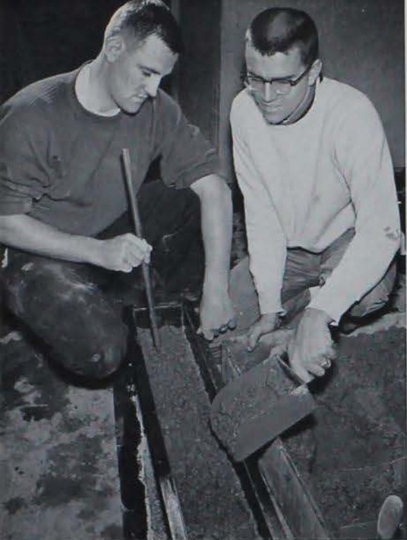
A few more shovels and they will have a perfect block of mud.
