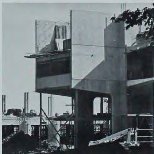
WORK IS WELL UNDERWAY on the Towers at the Poultry Farm destined to hold 1800 men.
