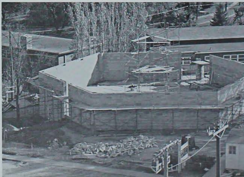
A LOT OF PUSH, a lot of power, and a lot of prayer made the building of the new chapel possible for University Lutheran.
