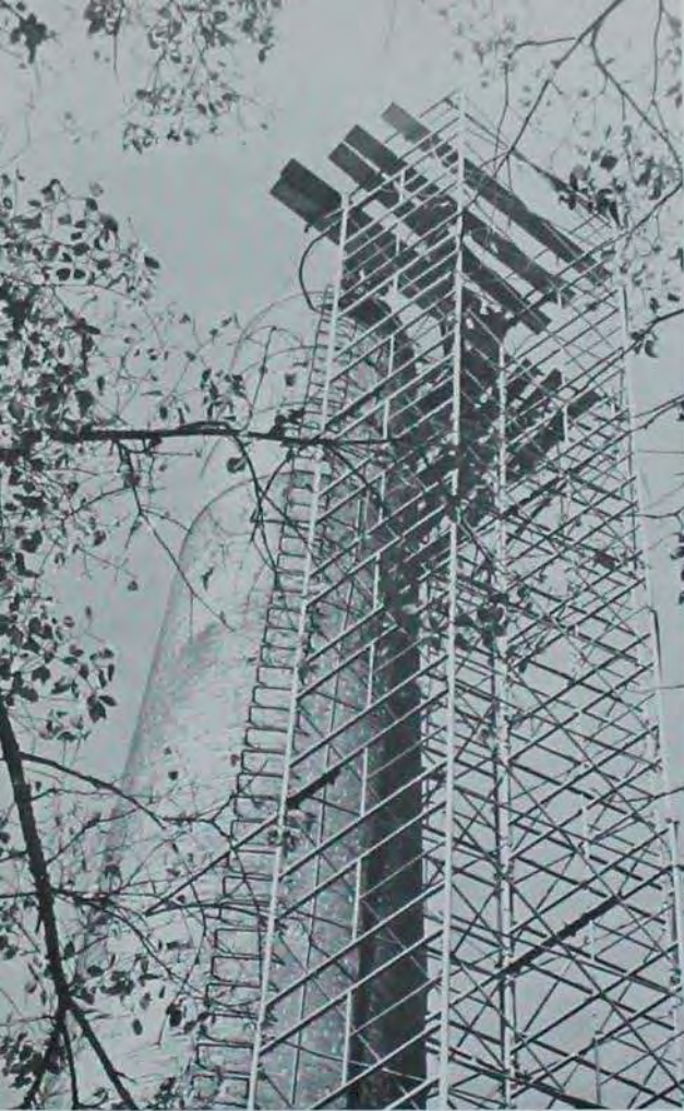
BUILT during the 1910's to provide an outlet for fumes from a boiler to run experimental equipment, the M.E. tower received a face-lifting when 30 feet of deteriorating brick were removed this fall.
