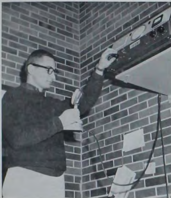
RADIO connections to the mobile unit are checked out by Edward Dunham. A quick call on this set will send the ambulatory clinic to wherever it's needed.
