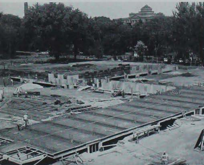
Increased student enrollment through the years has brought increased need for dormitory construction. The newest residence for men, Helser Hall, was built in 1957.
