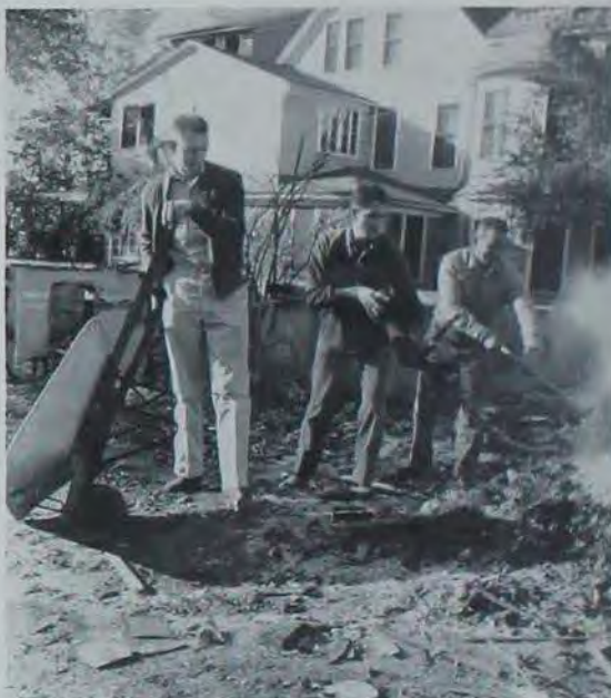
WITH THEIR OLD house torn down, Lambda Chi's pitched in with hopes of speeding up the construction of their new house.
