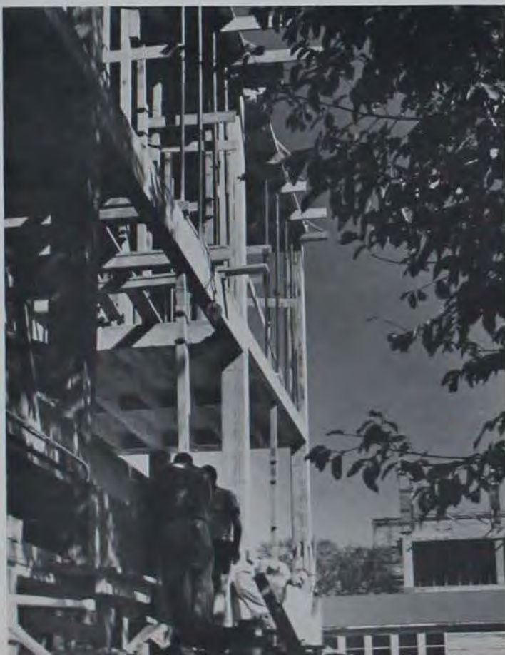
THESE WORKMEN are doing outside finishing on the south wall of the Service Building addition.
