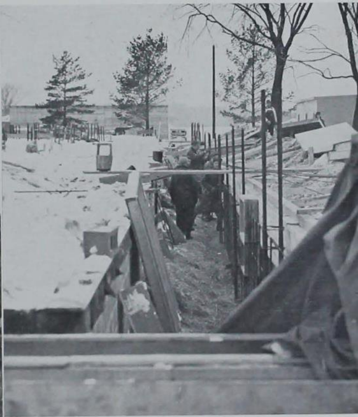
Work on the Electrical Engineering building goes on in spite of snow.
