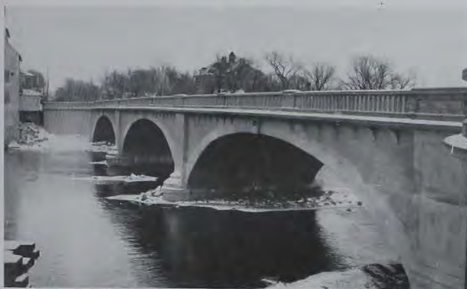
Bridge at Shellrock, Iowa. Designed, Supervised and Constructed by Alumni of Civil Engineering Department
