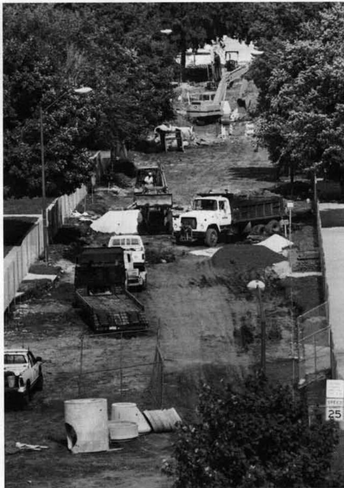
(Above) Work on Osborn Drive continues into the late summer, disrupting bus schedules and causing an inconvenience for those who remained on campus. The project was part of an effort to widen and resurface the road as well as install new control gates. This view of the project is looking east from the roof of the College of Design.
