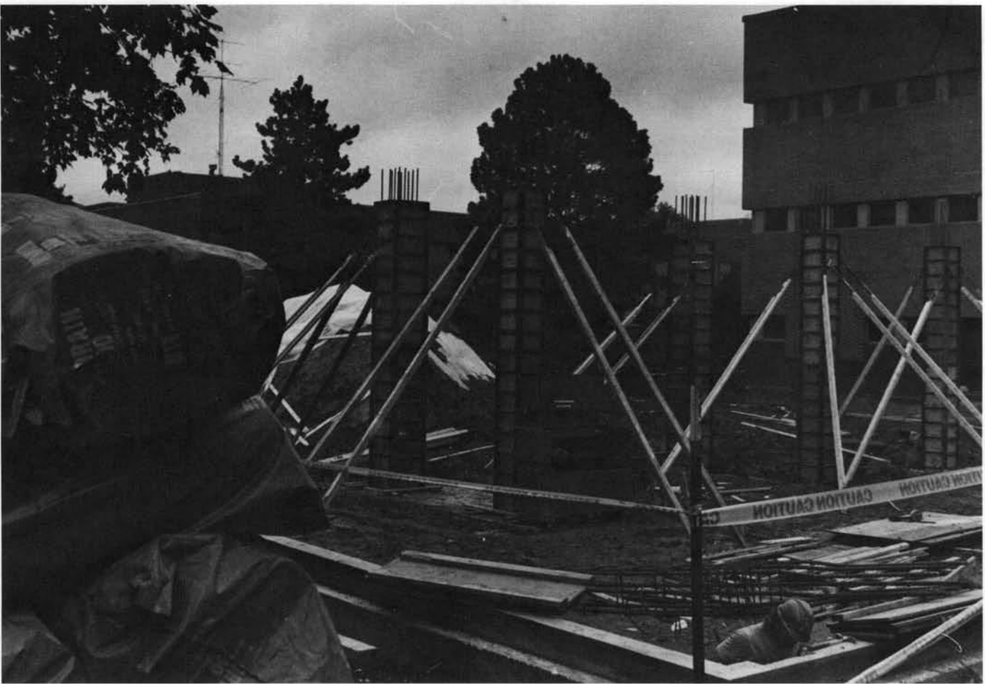
(Above) Workers begin work on the foundation of the $8 million, three-story addition to Sweeney Hall. The addition, which is slated for completion in December of 1993, will house new state-of-the-art laboratories for use by both faculty and students in the College of Engineering.
